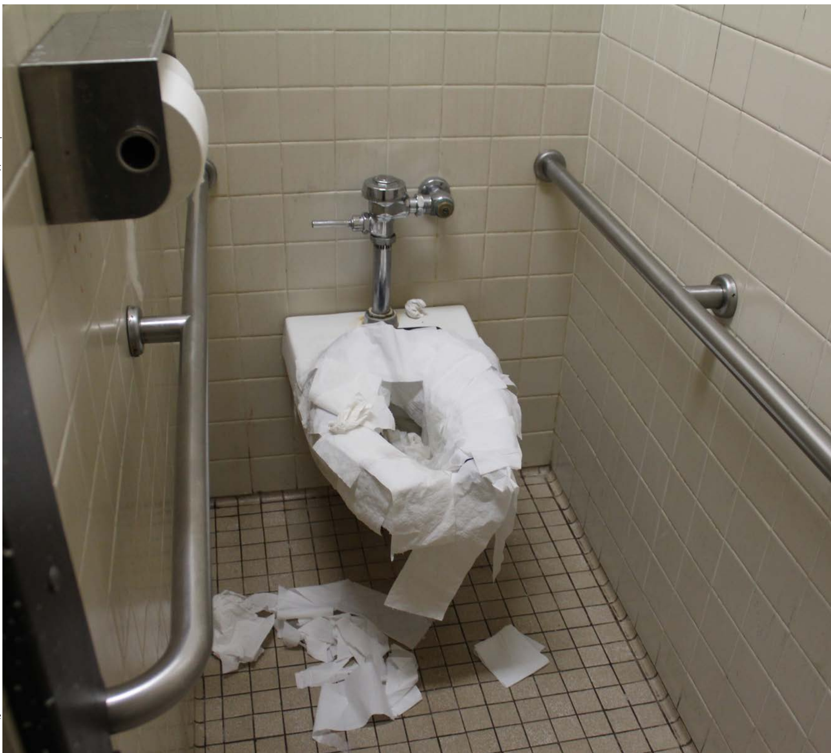
This toilet in the boy's bathroom, among others, has faced vandalism.
