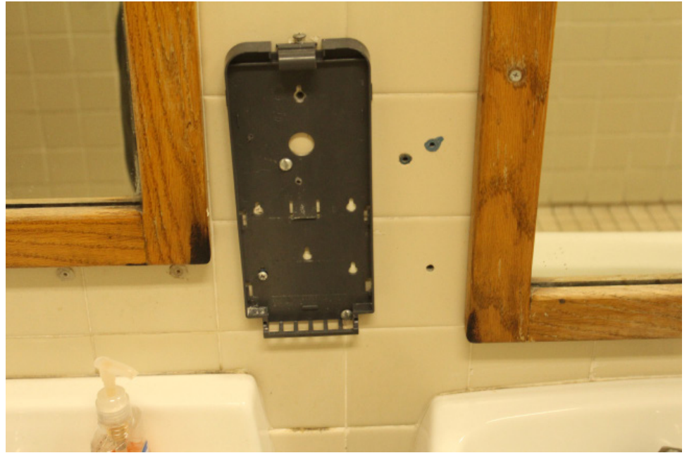
A soap dispenser torn off the wall in a Central bathroom. WHITMAN RUTLEDGE | The Register
