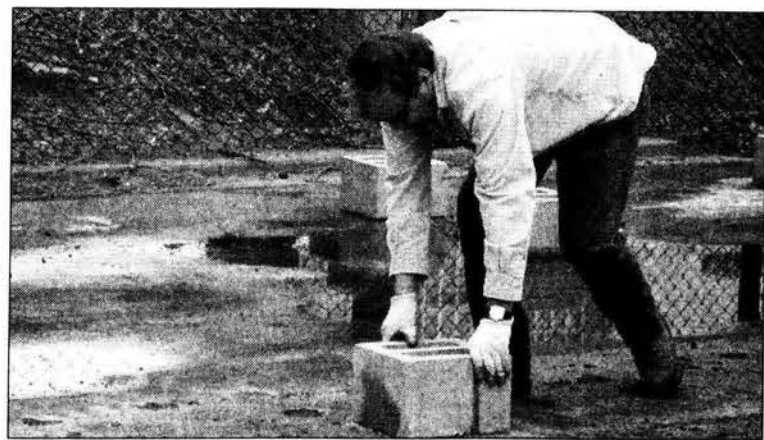
A worker sets up cinderblock bases for the portables to be set on. Central is receiving 25 portables.
