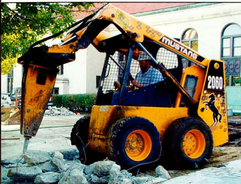
Below. Dennis Gentry, construction worker, breaks the ground of the West sidewalk to run wires to a new electrical transformer. PHOTO Quentin Lueninghoener
