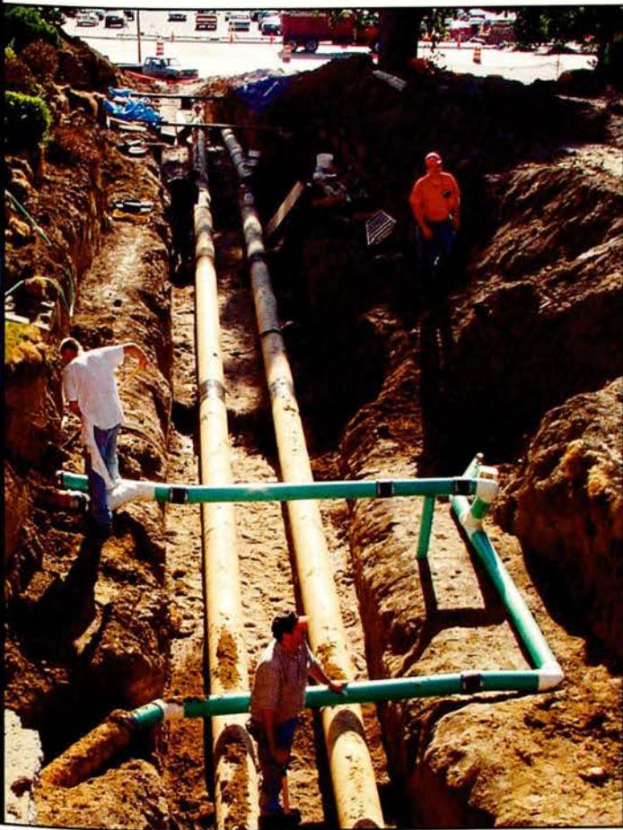
Below. Workers clear out a trench running by the South side of the school. The pipes will run hot and cold water for the air conditioning when it is installed. PHOTO Joe Meyer
