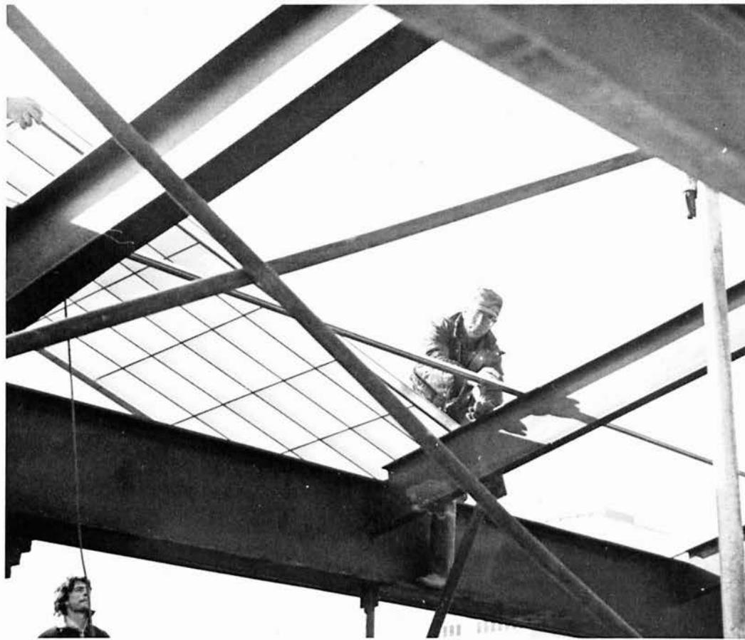
(Above right) The helicopter lowers beams on one of the hundred trips over the courtyard. Watch your step.
