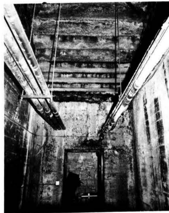
A subterranean view of Central's marble steps. Daylight can be seen peeking through the cracks when one is standing below.
