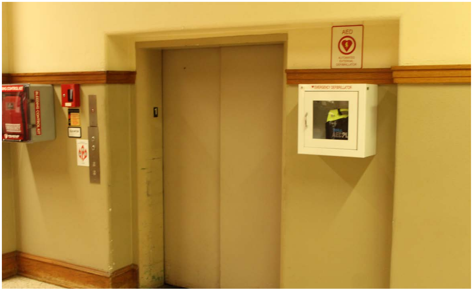
The main building elevator is often slow or broken. Photo courtesy of The Register
