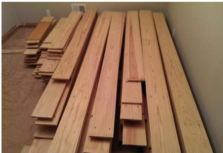
Step 3: The wood is stacked in Hamill's dining room while the initial flooring is removed.
