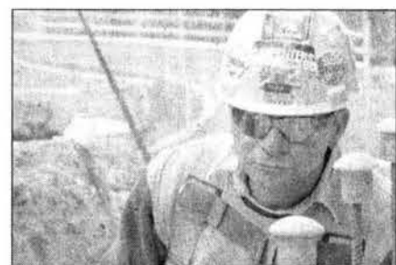
Here is a view of the field from a cafeteria window (middle). Travato places a blue chalk line for the stair structure (bottom right).
