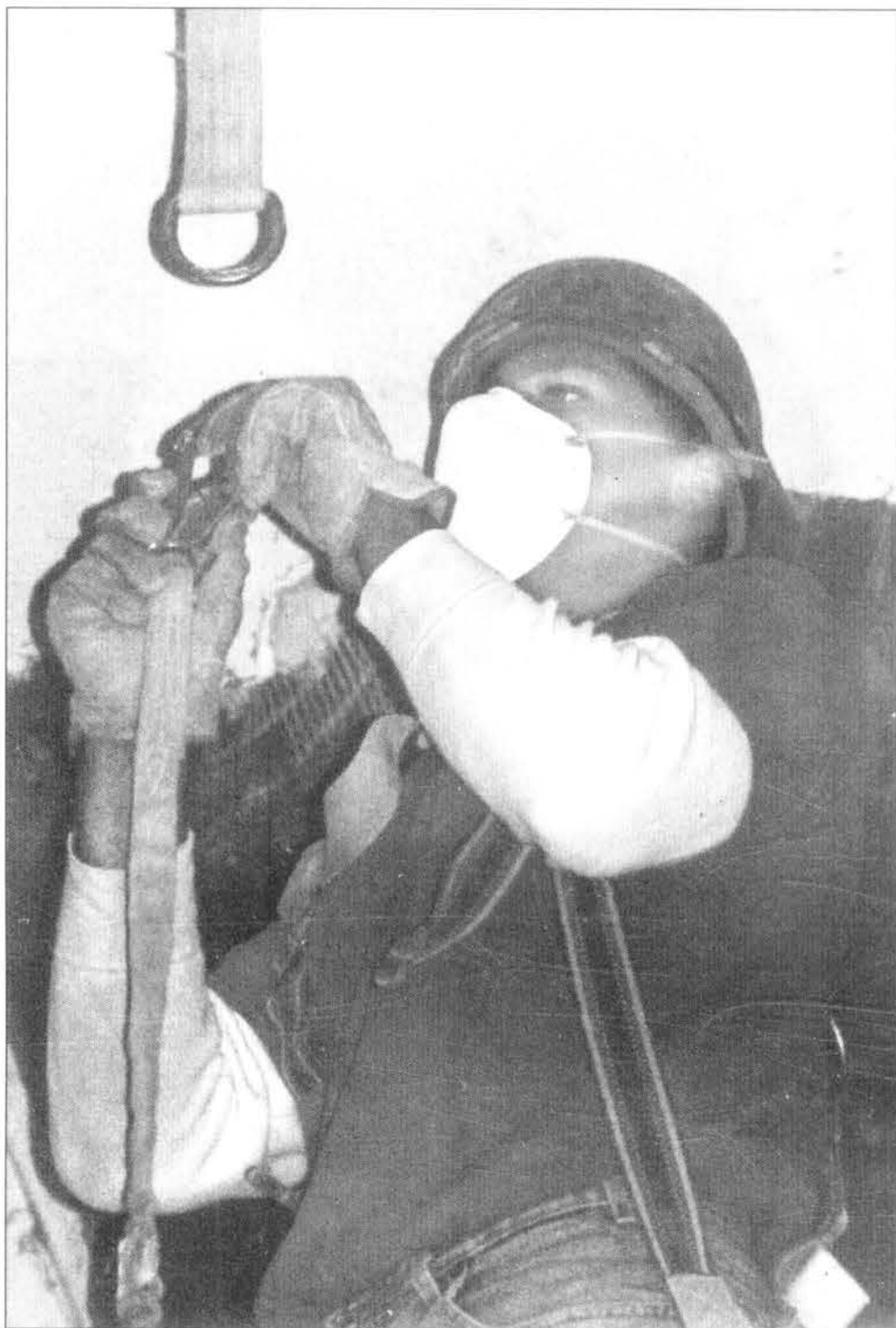
Photo by PAULA SALHANY/THE REGISTER Brian Barnes fastens his harness before removing old plaster from the ceiling in the physics rooms on the fourth floor. The work displaced the classes for several weeks and physics classes are still scattered throughout the building.
